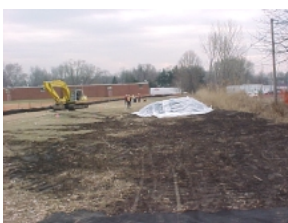
Soil is excavated and stockpiled for drying. The pile is covered to reduce dust.
