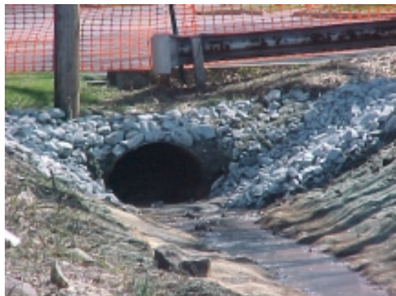
View of culvert at the terminus of W. Howcroft Avenue after restoration activities.
