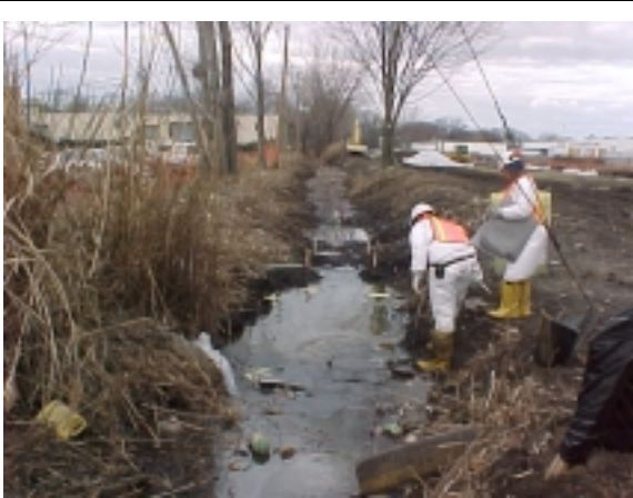
March 2, 2000 – View of the Swale looking West toward the Uniform Fashions Building.
