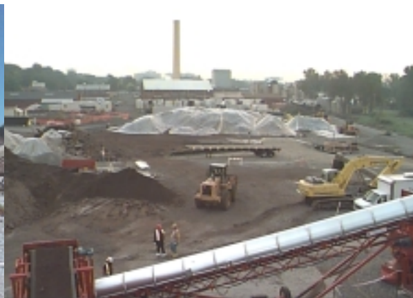
Behind shovel are processed soils. Feeder pile on left. Storage pile in rear, covered.
