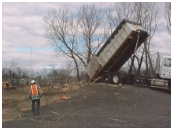
Roll-off containers were emptied using a ramp. Soil was stockpiled for off-site disposal.
