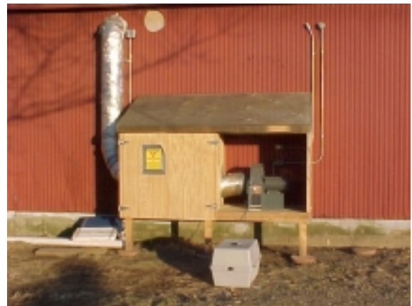
Exhaust fan and HEPA filter in rear of lab. Air monitor is stored in cat carrier for protection from elements.
