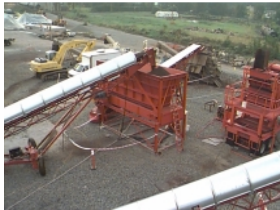
Separated soil feed into hopper to Thermo-Nutech SGS system for radiological sorting.
