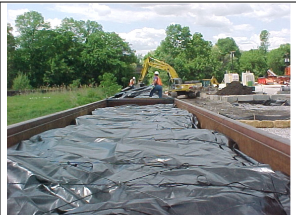
Railcar liner closed and secured and ready for shipment to Envirocare's facility in Utah for disposal.
