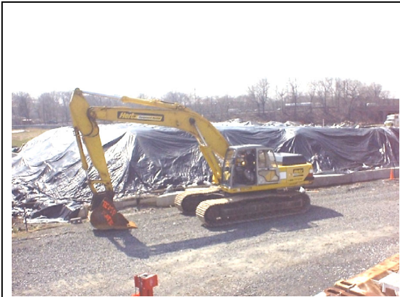
April 2001 – Covered soil stockpile before start of soil load-out. Excavator in foreground.
