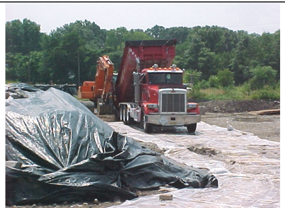
Unloading soil at MISS. Plastic liner was placed on the ground before unloading soil. Storage piles are covered with plastic to prevent wind erosion.
