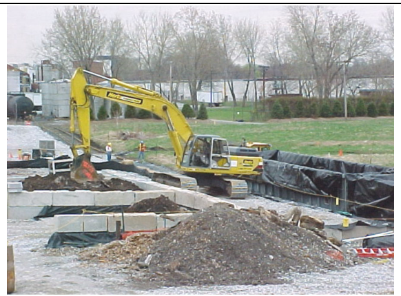
Excavator loading soil from the two storage bins into railcars containing liners.
