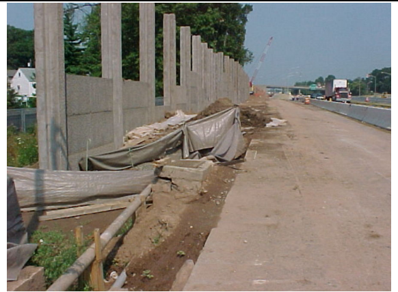
Interstate 80 – Erection of sound barriers. Excavated soil temporarily stored in work area.
