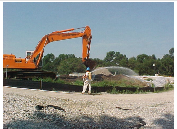
Excavation at MISS for water line installation. Worker spraying water for dust control.
