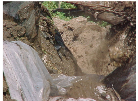
View of soil conditions found during trench excavation. Plastic had been previously placed on ground at MISS to prevent wind erosion.
