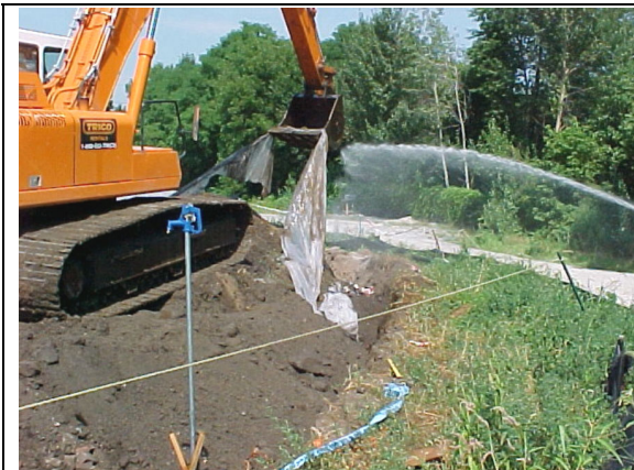
Excavation along access road perimeter at MISS for installation of water line and yard hydrants.
