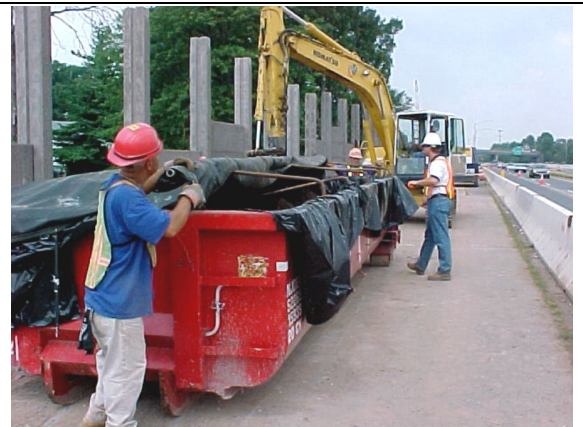
Workers closing liner before shipping container by truck to MISS for disposal.
