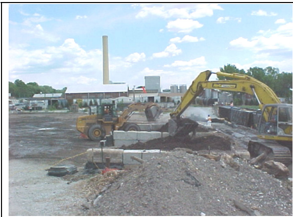
Soil being placed into storage bins by front-end loader. Excavator loading soil from bins into railcars.
