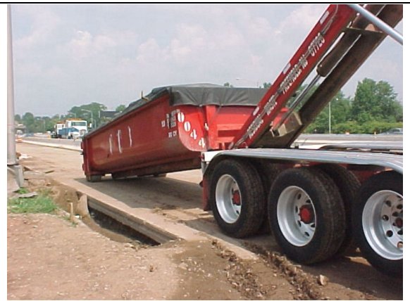
Delivery of roll-off containers for transporting excavated soil to MISS for disposal.
