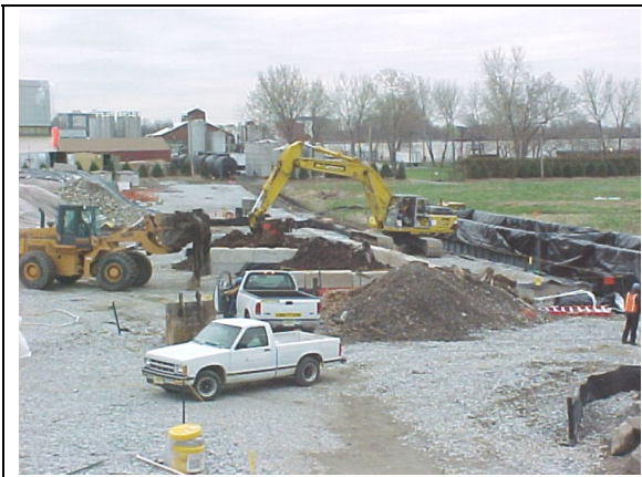
Front-end loader placing soil into storage bins. Excavator loading soil from bins into railcars.
