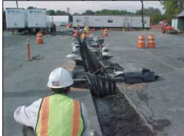
Laying geo-textile fabric and installing HDPE pipe. The SEC trailer and fabric structure are visible in the distance.
