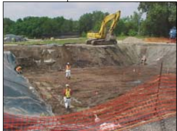
The dimensions of the excavated area was approximately 106 feet in length, 100 feet in width, and 11 feet (max) in depth.
