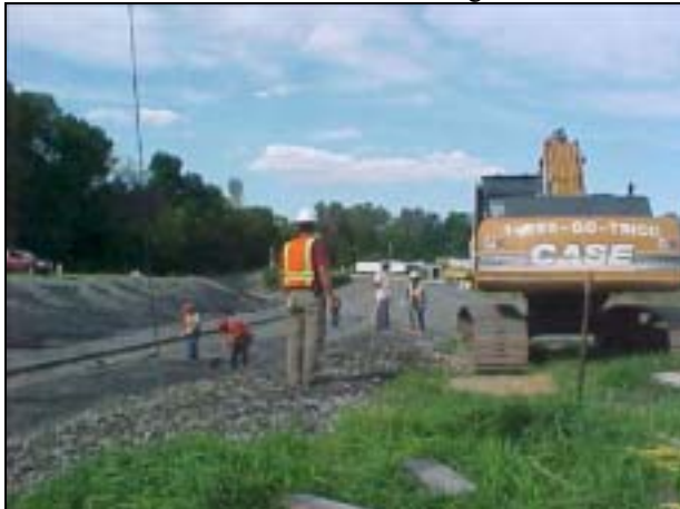
Workers spreading gravel adjacent to the Stepan Company railspur at the MISS. .
