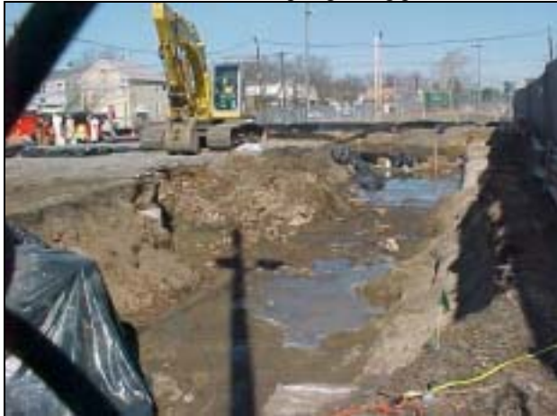
View from Rte. 46 looking North towards Kennedy Park. The exposed 3'x5' culvert is seen along the right (east).
