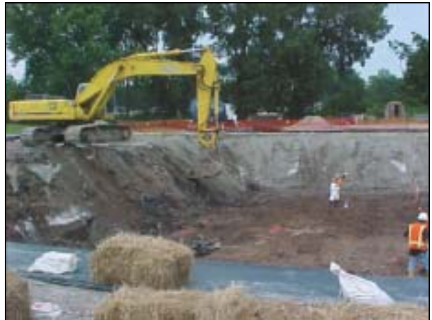
Hay bales were used to reduce storm water run-on and soil erosion during site preparation.
