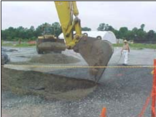
Start of excavation. Excavated soil is transported by front-end loader to fabric structure at MISS.
