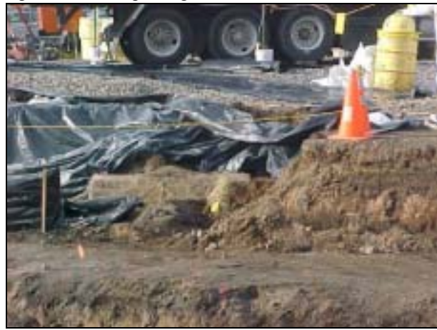
View from Sidney Street. Underground storage tank discovered during excavation at Cluster No. 1.
