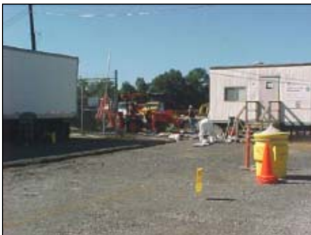
Sewer line entering the security gate at MISS. The grinder pump manhole is located to the left just past gate.
