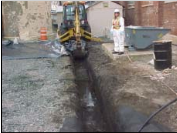
Trench excavation using backhoe between Stepan Company Buildings Nos. 4 and 67 adjacent to the stack.
