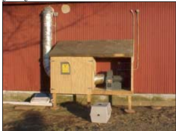
Exhaust fan and HEPA filter in rear of lab. Air monitor is stored in cat carrier for protection from elements.
