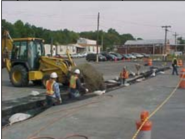
Front end loader placing "clean" fill in trench. The parking area for the FMSS trailers in the distance.
