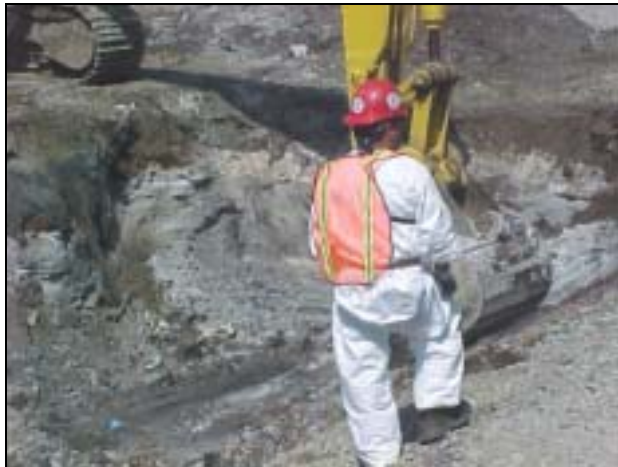
Excavation revealed the presence of white chalky deposits from former retention pond.
