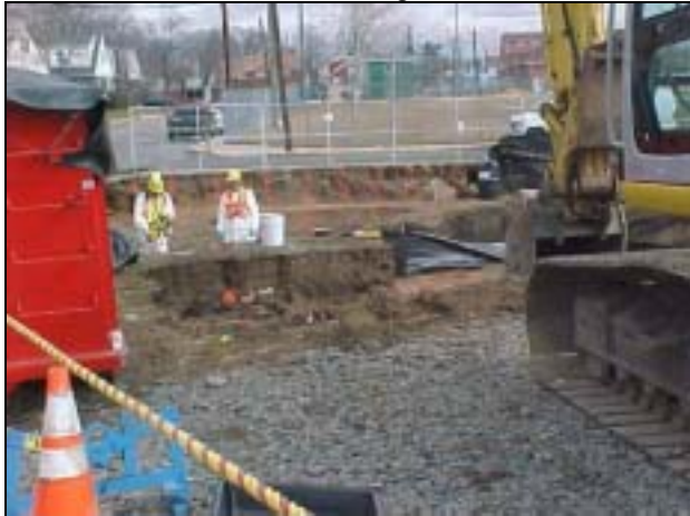
View towards Kennedy Park. Excavation visible adjacent to roll-off container. Soil sampling being performed.
