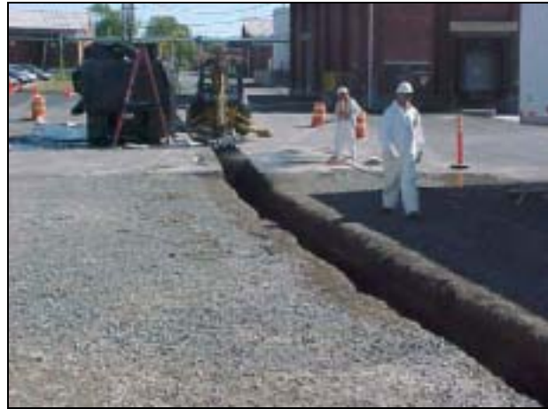
View of trench looking east toward Stepan Company's Building No. 67. Water spray being used in background.
