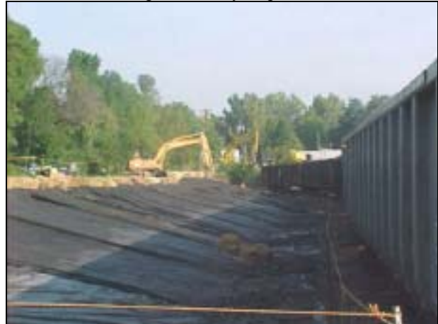
Removing soil along the rail spur for safer access to the cars.
