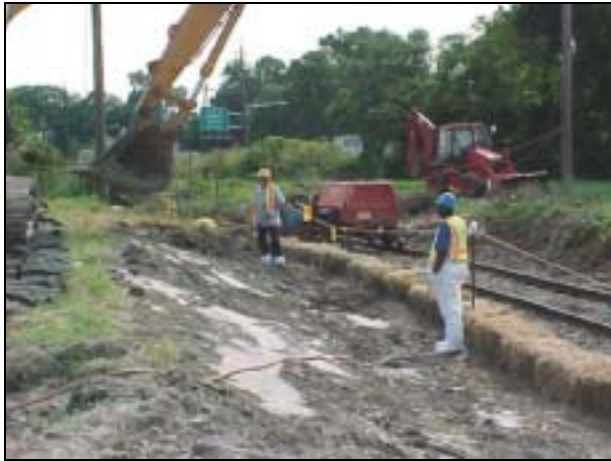
Excavator is removing soil to reduce the slope of the embankment for the rail banks along the railspur.
