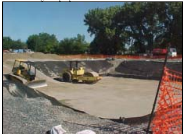
Roller used to compact the "clean" backfill material. Fill material was installed in lifts and compacted.
