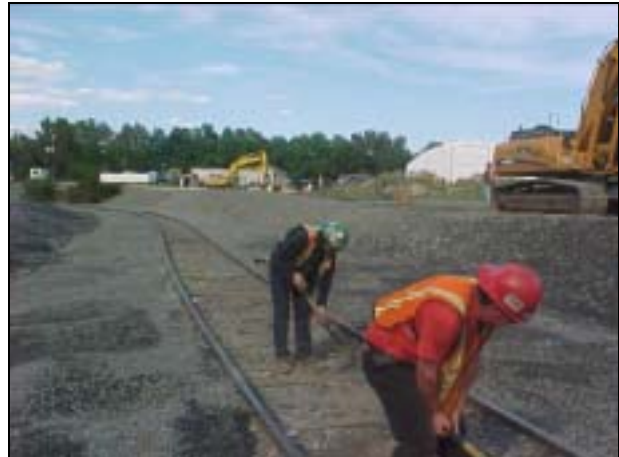
View of Sears railspur at the MISS upon completion of slope cutback.
