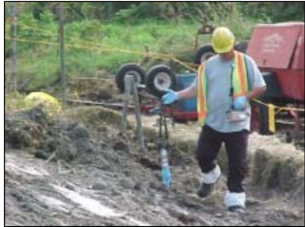
Gamma scans indicated elevated radiological readings for excavated soil generated by slope cutback.
