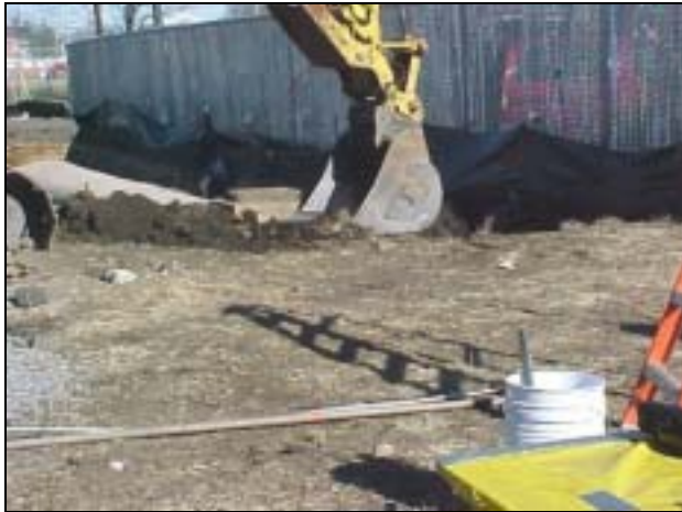
Excavator removing overburden on culvert. Exposed culvert shown near fence in background.
