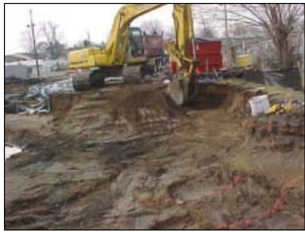
Looking south toward Rt. 46. Money Street is on the right. Excavator placing soil into roll-off container.
