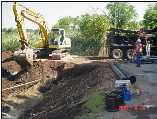
An excavator loads soil into a lined dump truck for transport to MISS for disposal.
