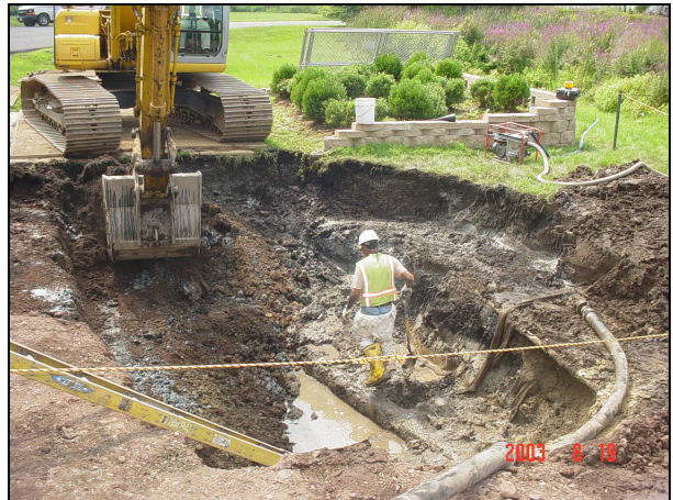
An excavator removes soil to expose the ruptured section of the water line.
