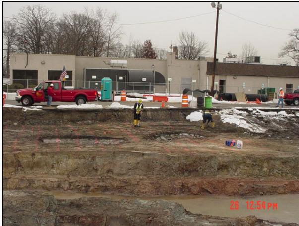
Accumulation of ground water in excavation at 160-174 Street properties.
