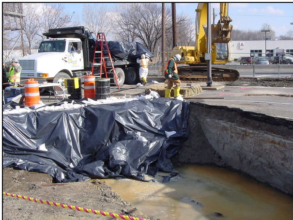
Plastic sheeting is used to cover the contaminated "face" of excavation at the end of the work day.
