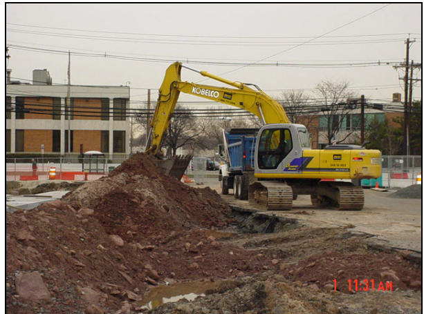
An excavator removing soil from the parking areas and loading into dump trucks for transport to the MISS.
