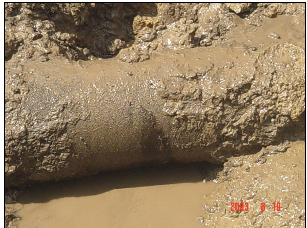
The excavation reveals the broken section of the water line.
