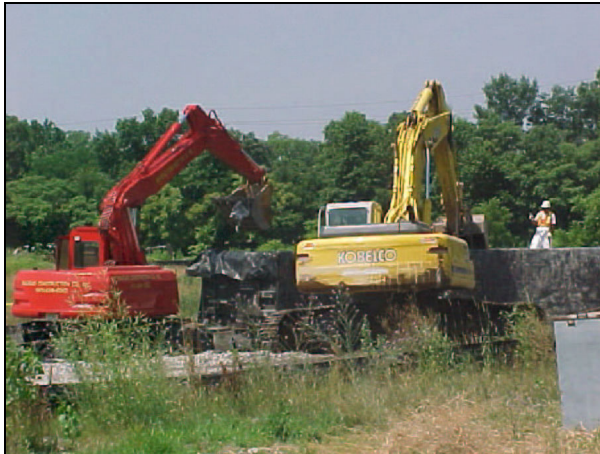
Excavators loading soil into rail cars from storage bins for shipment to off-site disposal facility.
