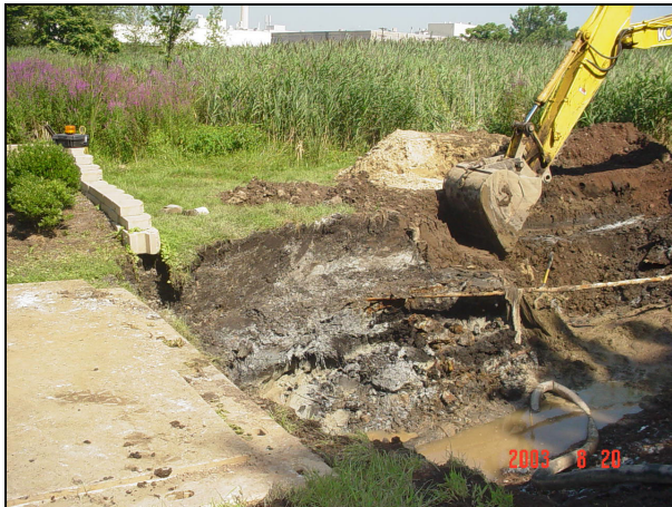
Excavation to repair the second rupture of the water line at 149-151 Maywood Avenue during August 2003.
