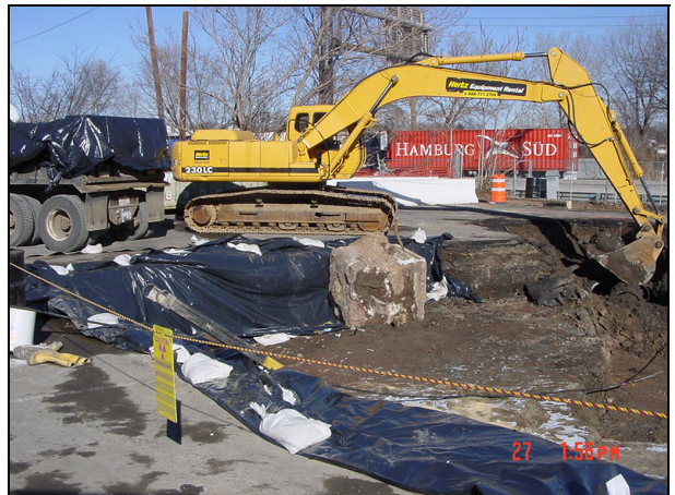
The excavated soil is loaded into lined dump trucks for transport to the MISS for disposal.
