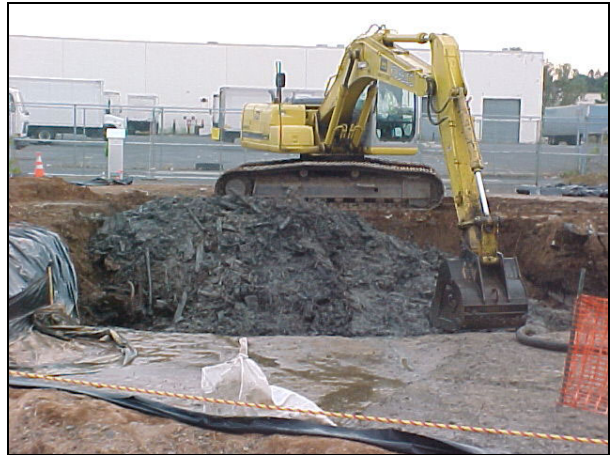
Additional excavation being performed at the property. Significant amounts of debris was found in the soil.
