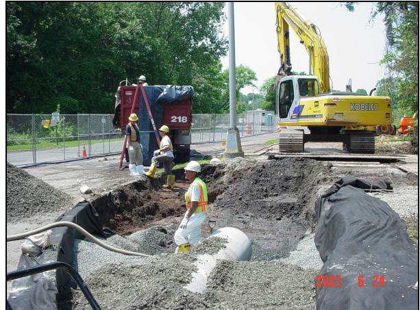
Pipe bedding and structural fill was placed around the new section of drainage pipe.
