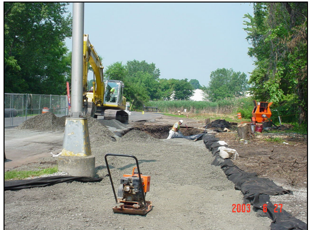
Backfilling and compaction of the pipe bedding and structural fill is being performed.
