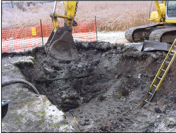
Excavation to repair broken water line at the 149-151 Maywood property during January , 2003
