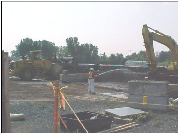
Excavator removing soil from load-out bins and placing into rail cars. Water spray used for dust control.
