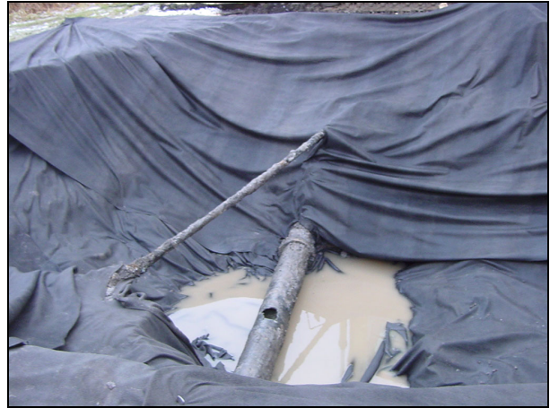
The ruptured water line has been isolated and the excavation covered with geo-textile fabric.
