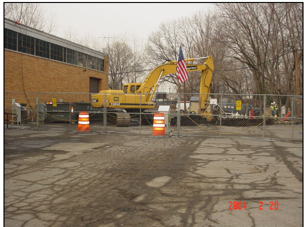
Excavation being performed in the parking areas on the north side of the building.
