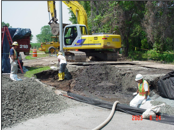
An excavator was used to remove the soil for installation of the concrete drainage pipe.
