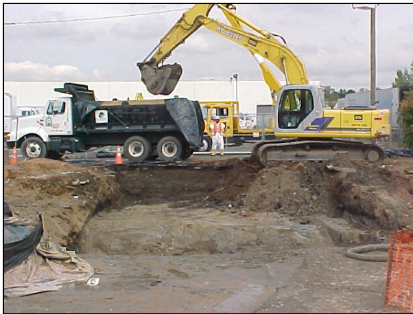
An excavator is used to load soil into lined dump trucks for transport to the MISS for disposal.
