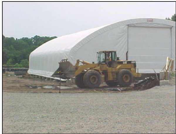
Front-end loader is use to transport soil from inside fabric structure to load-out bins near rail cars.
