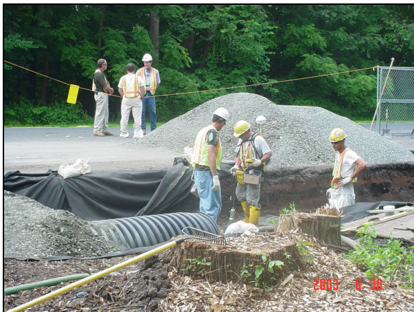
Installation of HDPE pipe sections. Tree clearing was performed prior to excavation..
