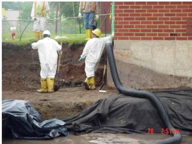
Excavation performed along building. A hose was used to direct water from roof drains away from the excavation.
