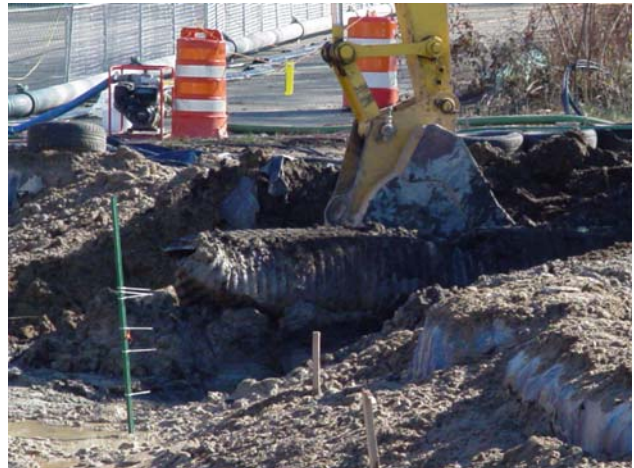
An excavator is used to remove an old drainage pipe on the property.
