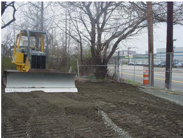
A bulldozer is grading the top soil to establish the final grade.
