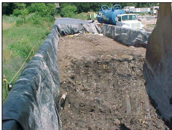
View of partially loaded rail car. When full, the liner will be closed and tied to prevent soil loss during shipping.
