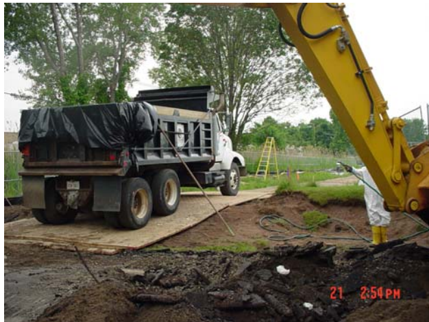
The excavated soil was placed into a lined dump truck for transport to the MISS.
