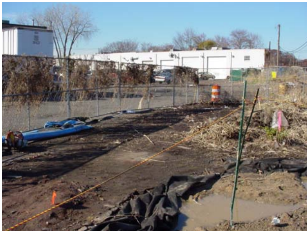
An access road for the dump trucks was prepared to facilitate the transport of excavated soil to the MISS.
