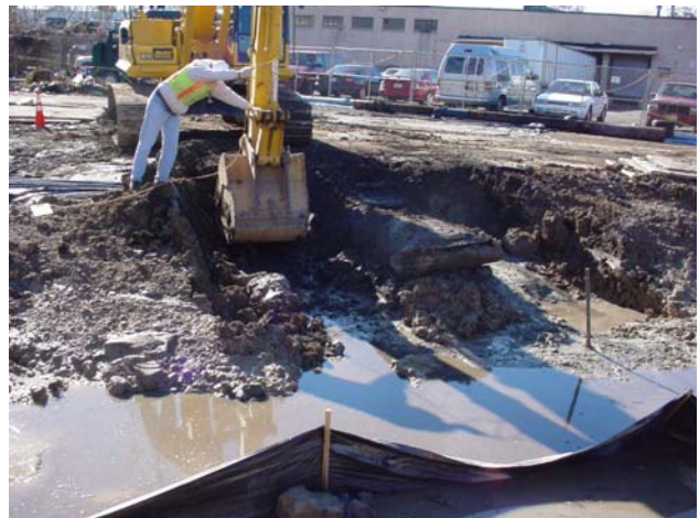
Accumulated water in the excavation is pumped to a fractionalization tank for subsequent transport to MISS.
