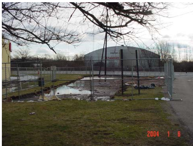
Excavation was also performed to remediate an adjacent area of radiologically contaminated soil.
