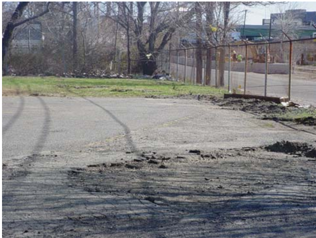
Initial conditions at the property located at 170 Gregg Street showing damaged asphalt parking lot.
