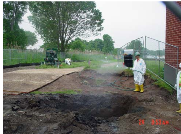
Water is sprayed at the excavation site to prevent airborne dust emissions.
