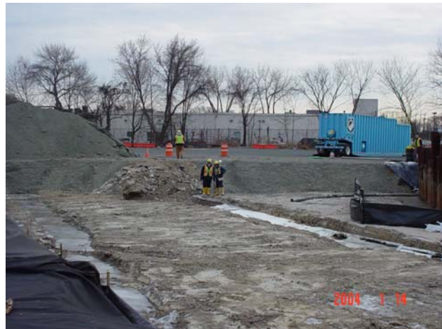
Debris is visible from excavation. A vibrating screen was used at the MISS to remove debris from the soil.
