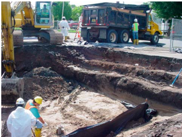
The excavated soil was placed into a lined dump truck for transport to the MISS for disposal.
