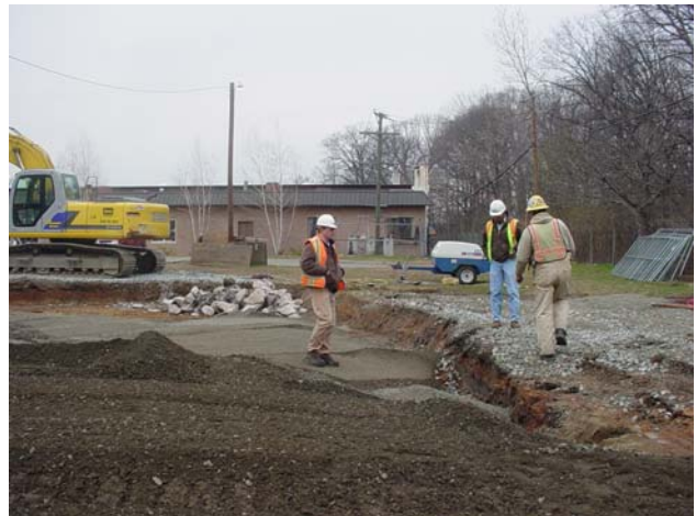
Backfilling activities including the compaction of the structural fill and placement of top soil.
