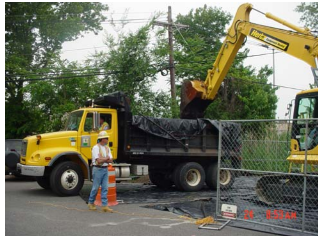
The excavated soil is transported to the MISS and subsequently loaded into rail cars for off-site disposal.
