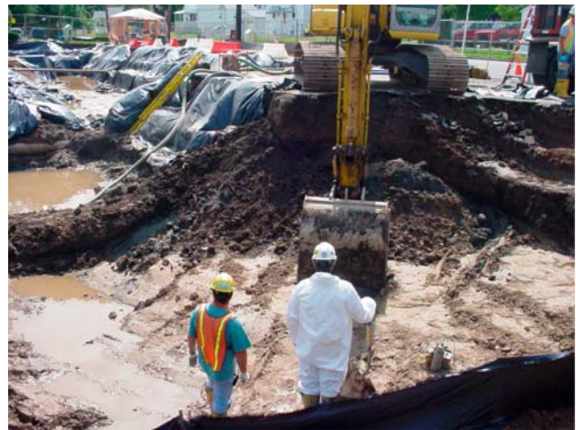
Accumulated water in the excavation is pumped to an on-site fractionalization tank for transport to MISS
