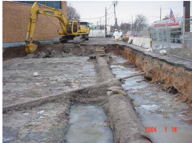
Excavation being performed with the storm water line and electrical conduit exposed.
