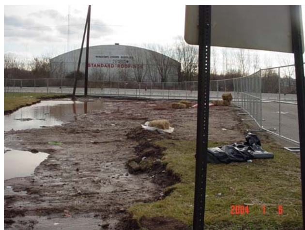
Temporary fencing was erected to establish the controlled access area during excavation and backfilling activities.
