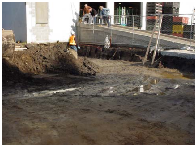
Removal of the concrete stairs to facilitate remediation of impacted soils adjacent to the building's ramp.
