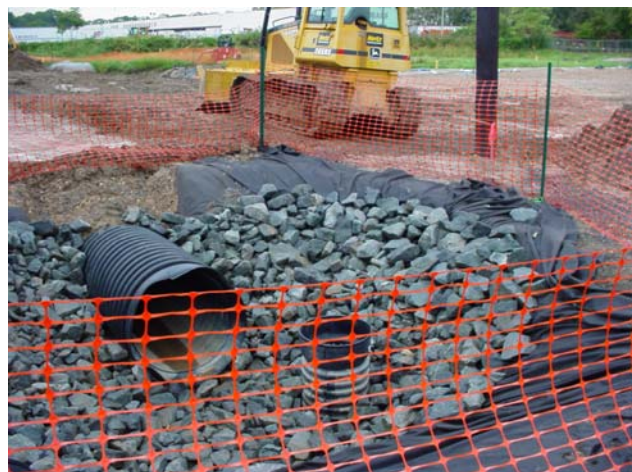
Completion of the temporary drainage basin. The bypass line will be removed upon completion of the remediation.
