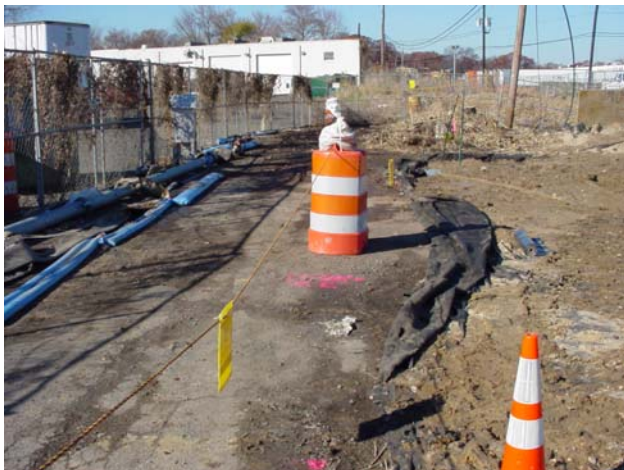
Plastic bladders filled with water were placed along the perimeter of the excavation to divert surface water run-on.
