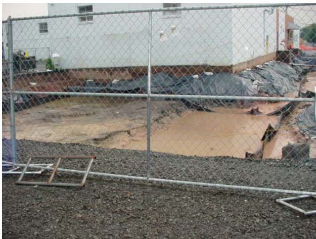
Fencing was erected at the property boundary to establish the access control area.
