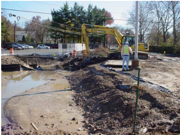
Excavation of former open channel culvert at the property located at 85-103 NJ RT. 17 South.
