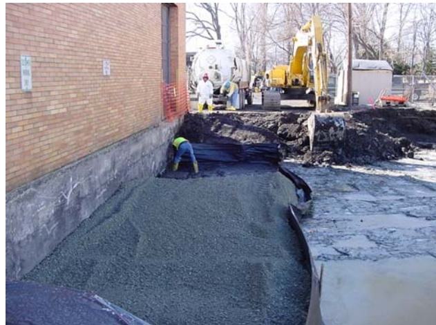
Backfilling along the building foundation on the north side of the building.
