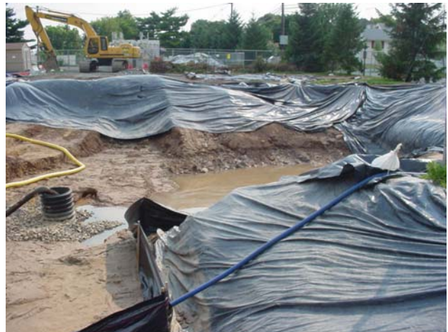
Polyethylene sheets were used to cover the impacted soils surrounding the temporary drain.
