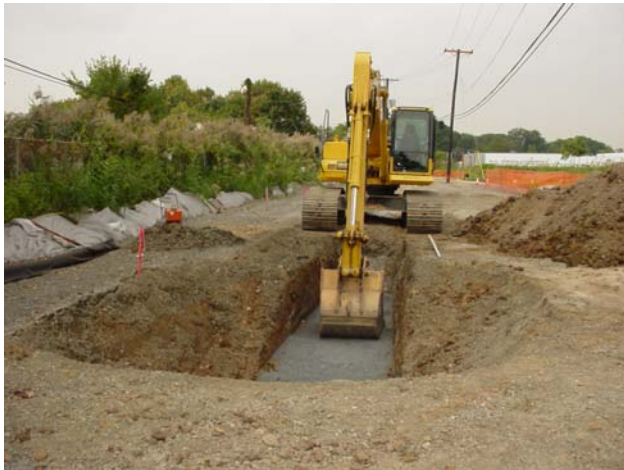
Excavation at the 149-151 Maywood Avenue property to install by-pass line for open channel remediation.
