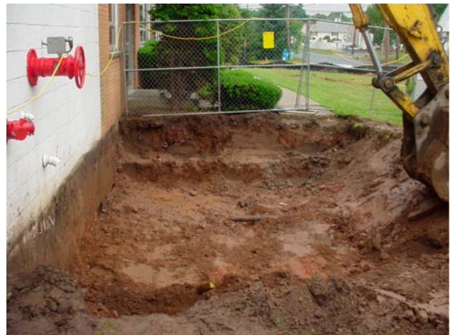
Additional excavation was performed along the building on the Hancock Street side.
