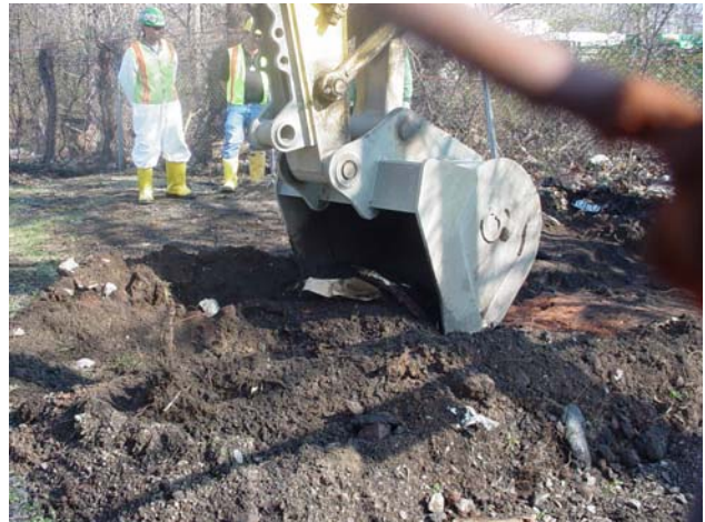
An excavator is removing the radiologically contaminated soil for transport to MISS.
