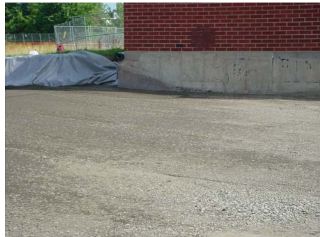
Establishment of the final rough grade at the site as part of the restoration process.
