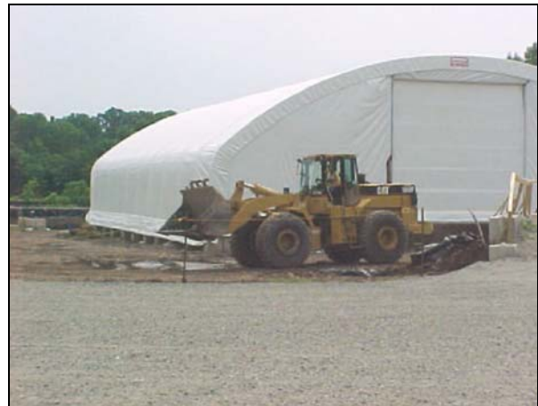
Front-end loader is use to transport soil from inside fabric structure to load-out bins near rail cars.
