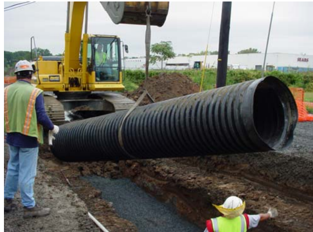
An excavator is used to install by-pass line section in the trench.
