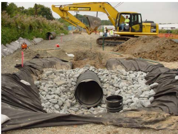
Construction of the temporary drainage basin. The excavator is covering the pipe sections with fill material.
