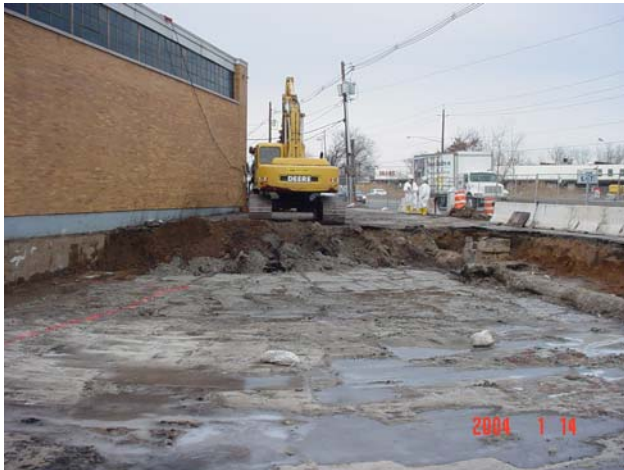
Excavation being performed at the east side of the building located at the 200 NJ Rt. 17 South property.
