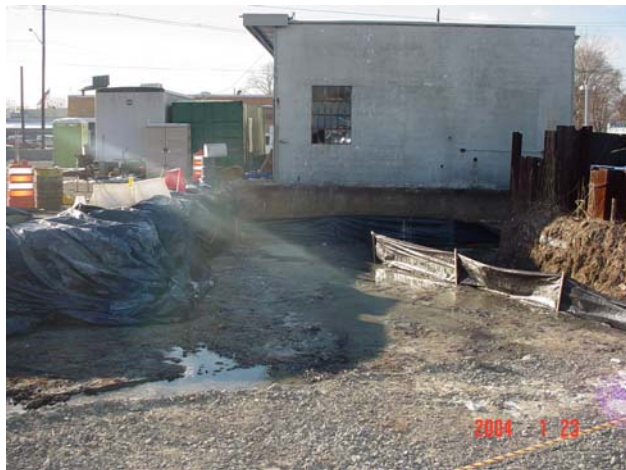
Backfilling in progress with the placement of structural fill in the excavation.
