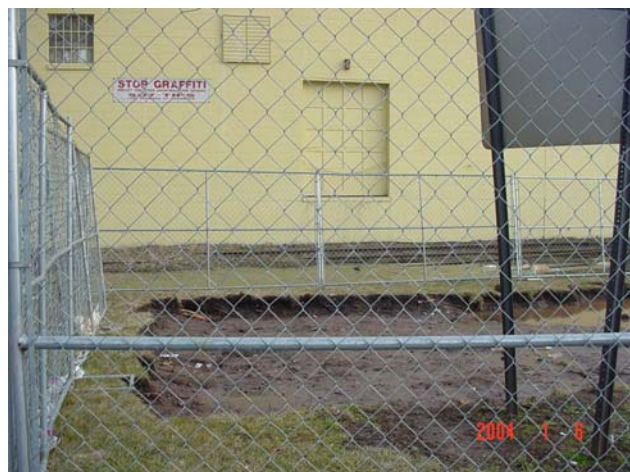
The depth of the excavation was shallow since only surface contamination was found.
