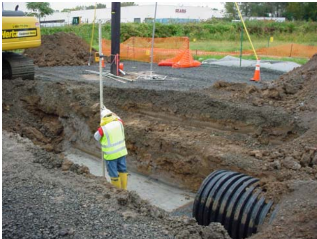
Establishing grade for the installation of the next section of the bypass line.
