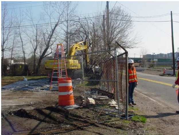
An excavator removing radiologically contaminated soil near the property boundary along Gregg Street.
