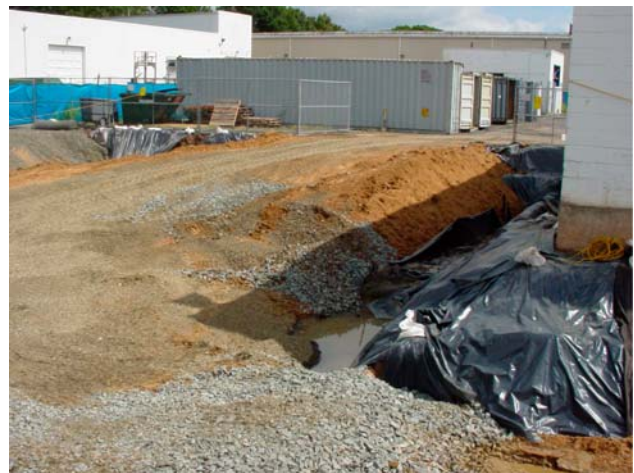
Backfilling partially completed; poly sheets were used to cover inaccessible impacted soils along the building.
