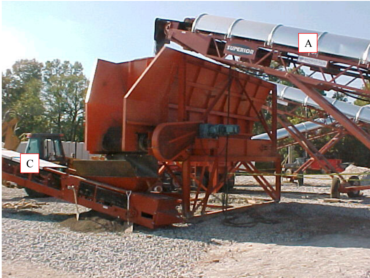
Surge Hopper to Maintain a Continuous Feed to the Radiological Sorting System
