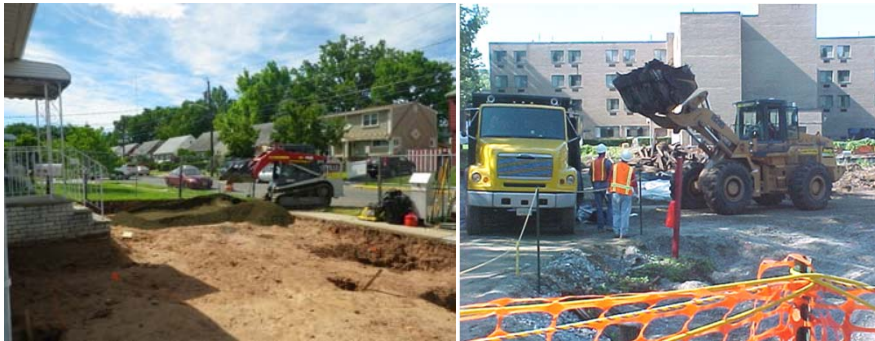
FUSRAP remedial actions at a Lodi, NJ residential property and at a health care facility in Rochelle Park, NJ. Note the workers are dressed in standard construction clothing.
