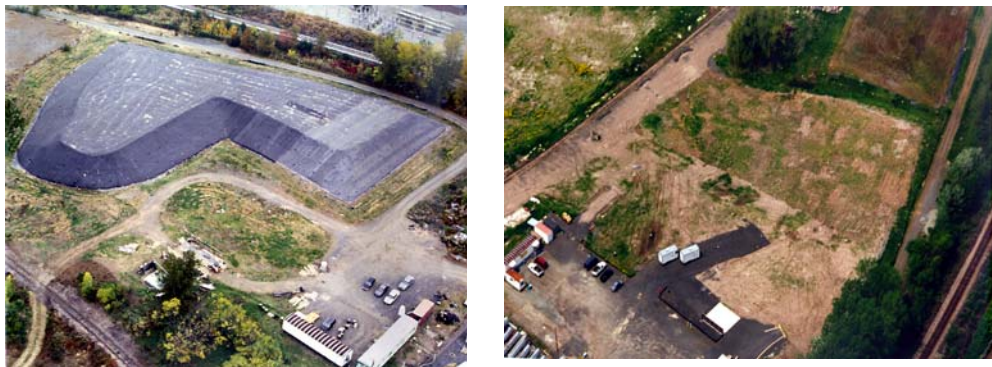
The MISS before (left) and after removal of the soil storage pile. The pile is in the upper portion of the photo on left.
