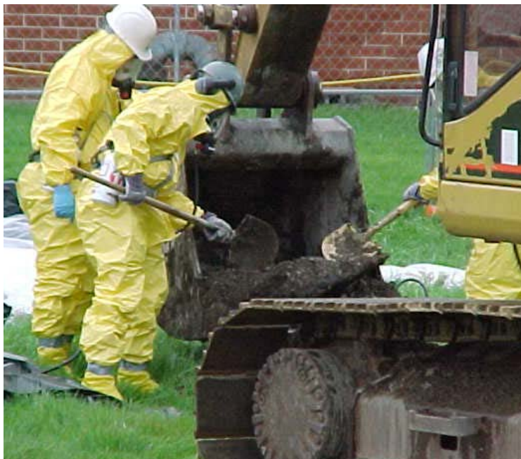
Workers in protective clothing uncovering a buried metal object at a Maywood property.
