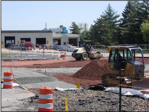
The NJ motor vehicle inspection station at Lodi (background) is in full operation as cleanup excavations move forward.
